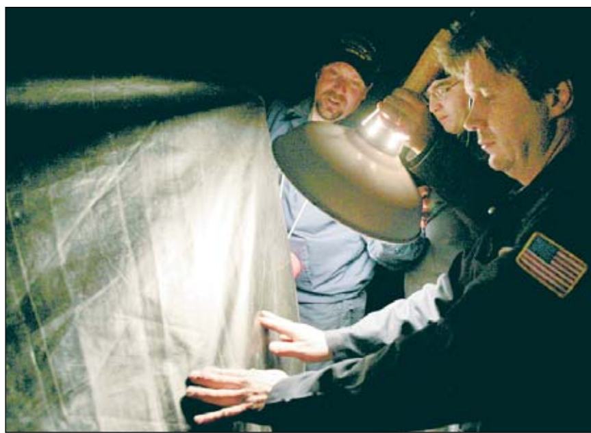
At bottom left, Charlie Shankle (from left), Tom McEwen and Tim Cartell shine a light on the envelope and use a walkie-talkie to check with a co-worker on the other side looking for tiny holes.
