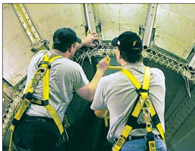
Brian Hershberger (left) and Rob Delagrance check the lacing at the metal nose cone where 16 battens come together to support the blimp.
